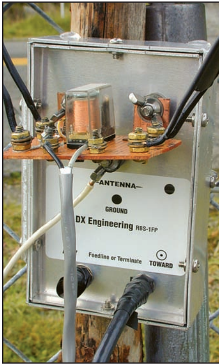
Figure 7 — The relay board is installed directly on the RBS-1 antenna terminals under a rain shield.
